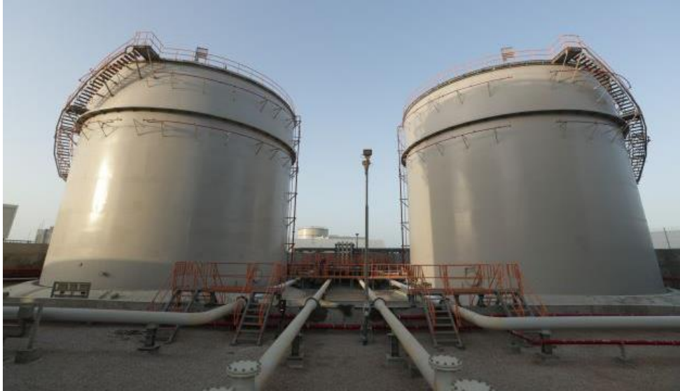
Fig. 2.12. General view of bunker fuel storage [57].
