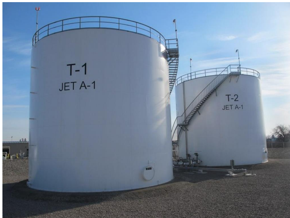
Fig. 2.5. Storage tanks for Jet A-1 [45].
