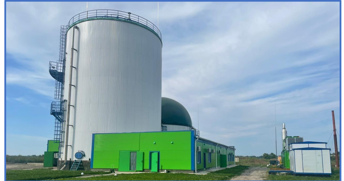
Dionis biogas plant – 20 000 m 3 /d
