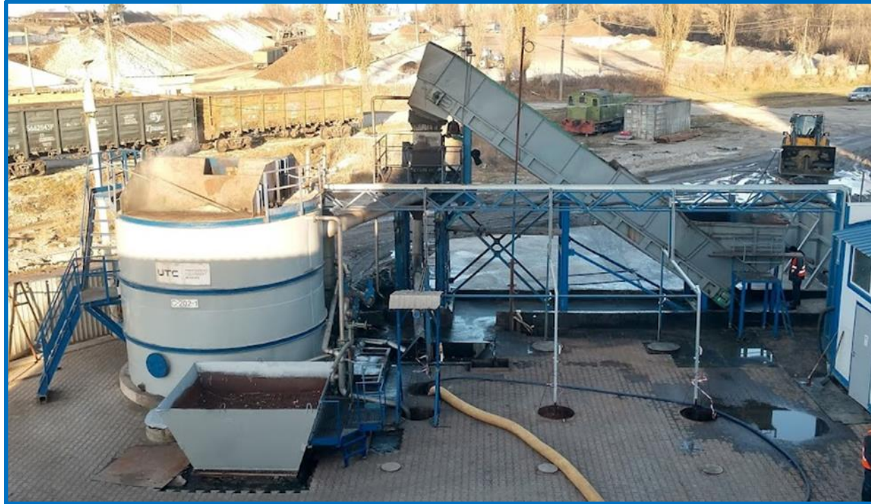
Wet milling system, mixing and pumping
