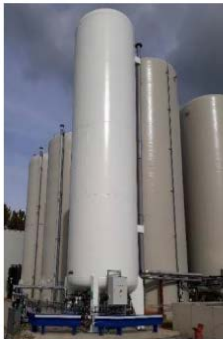
Vertical CO 2 Storage
