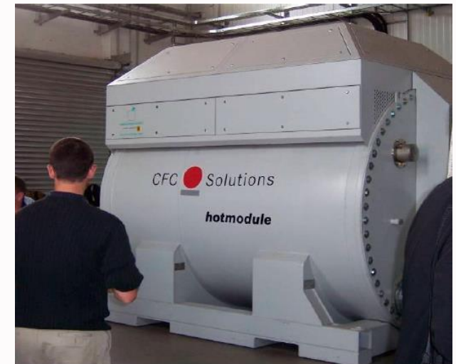
Molten Carbonate Fuel Cell (MCFC) for biogas in Leonberg, Germany (Source: Rutz)
