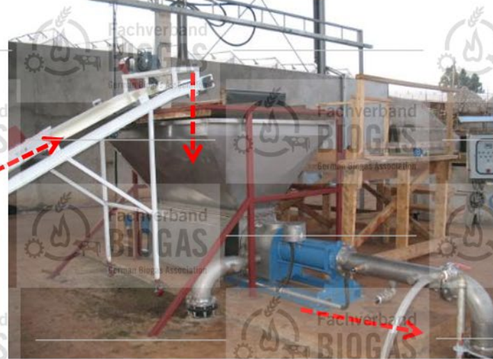
Dosing station with eccentric screw pump
