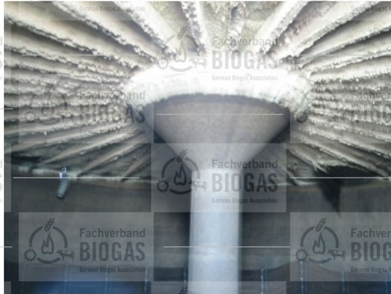
Sulphur deposits in the digester
